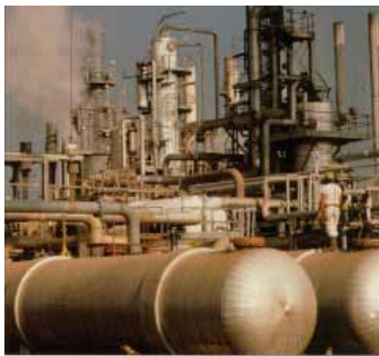
Pressure vessels used in the hydrocarbon processing industry represent the single largest application of roll-bonded clad plate.
